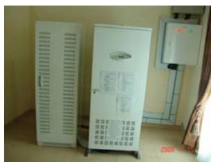
Equipment damage Citirahman Hospital
