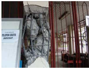
Compressive failure of RC column
