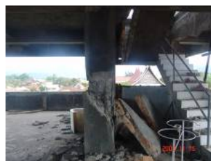
Structural damage, Selaguri hospital
