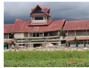
The Padang city bus terminal totally collapsed
