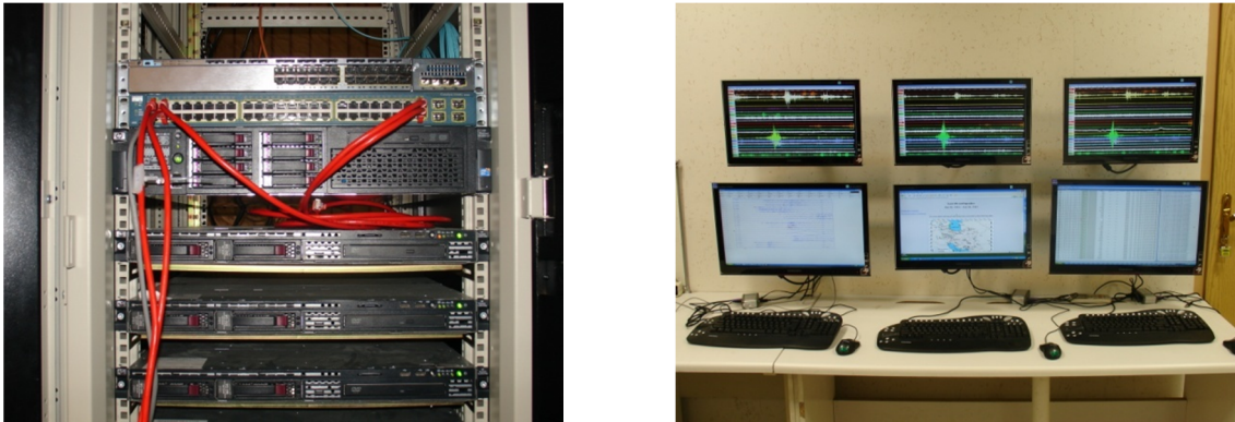
Figure 2. Computer rack and monitors in data acquisition center of IIEES.
