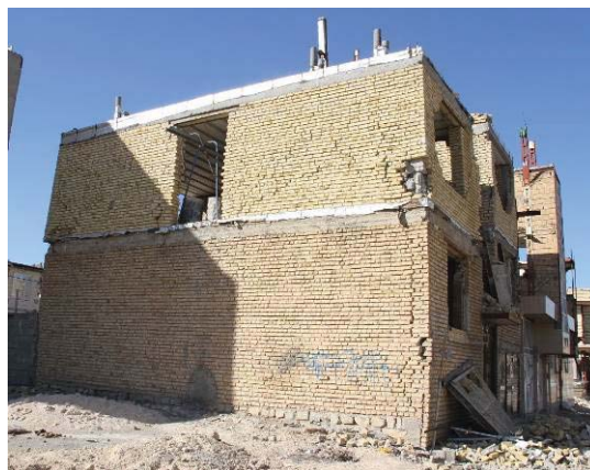
Figure 1. Inadequacy of the code provisions for confined masonry.
