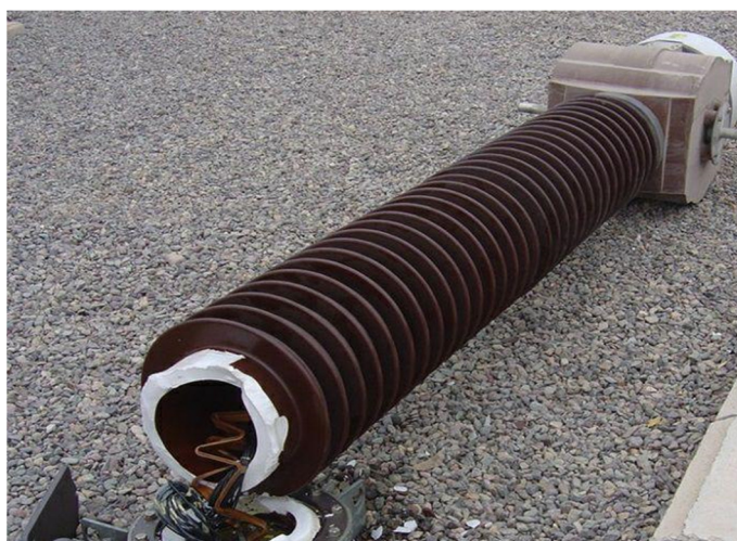
Figure 1. Failure of porcelain insulators in high voltage substations (Khalvati, 2008).
