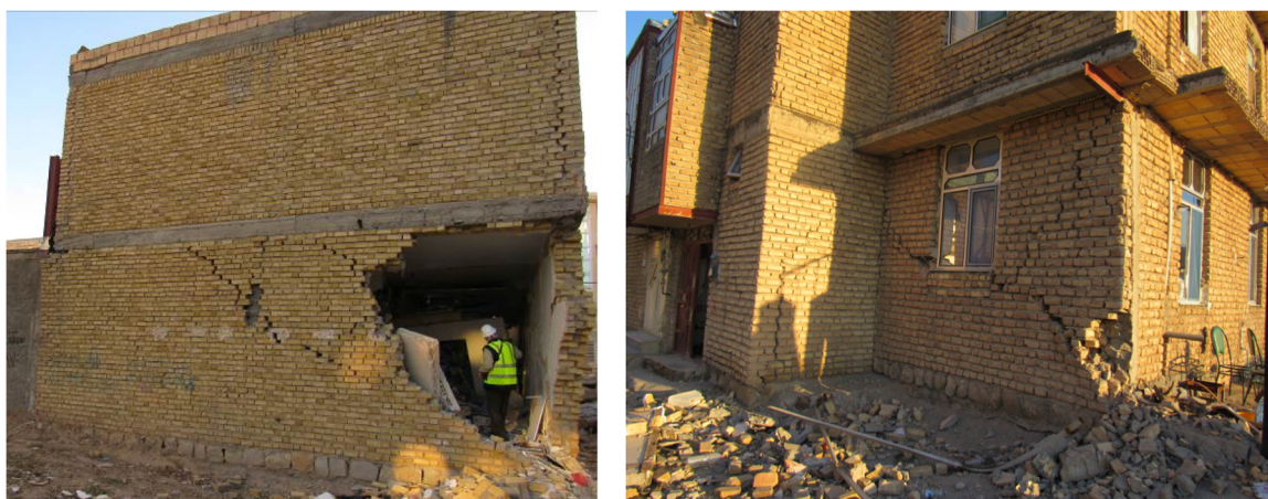
Figure 1. Observed damages in URM walls in Sarpol-e Zahab earthquake.
