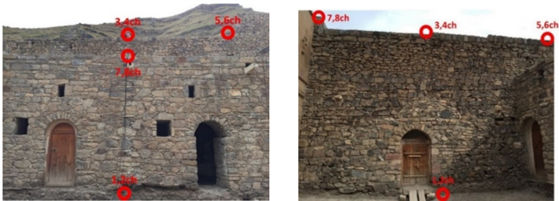
Figure 2. Position of sensors for the northern wall (Case 4) (Left) and the eastern wall (Case 5) (Right).
