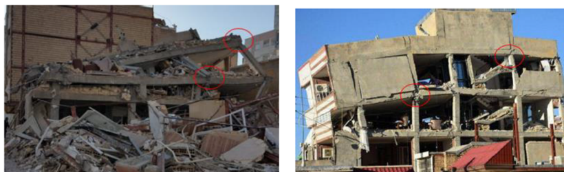
Figure 1. Collapse of the RC buildings due to the failure of beam-column connections in recent earthquake (12 November 2017) in Kermanshah-Iran with magnitude of 7.3.
