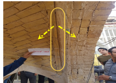
Figure 4. Opening between the vault and the rib cover in the unreinforced structure.
