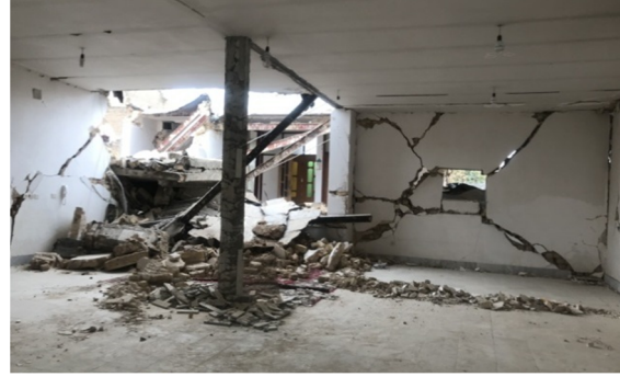
Figure 2. Damaged walls and roofs.
