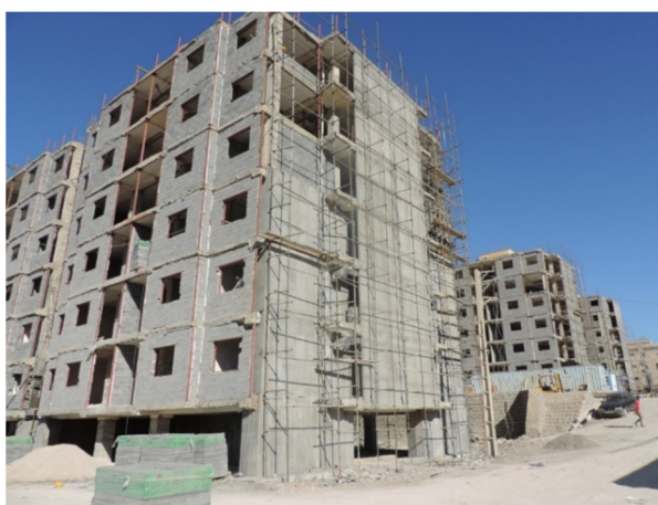
Figure 1. concrete structure having a shear wall in one direction and a moment resisting frame in another.
