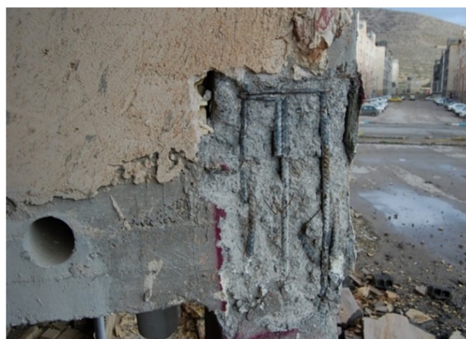
Figure 2. Lack of sufficient stirrups in columns.
